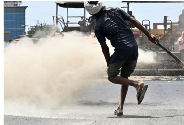
Hellfire: A road worker, braving the heat and dust, repairing a damaged road in Palayamkottai, Tirunelveli on July 9. SHAIKHMOHIDEEN. A
