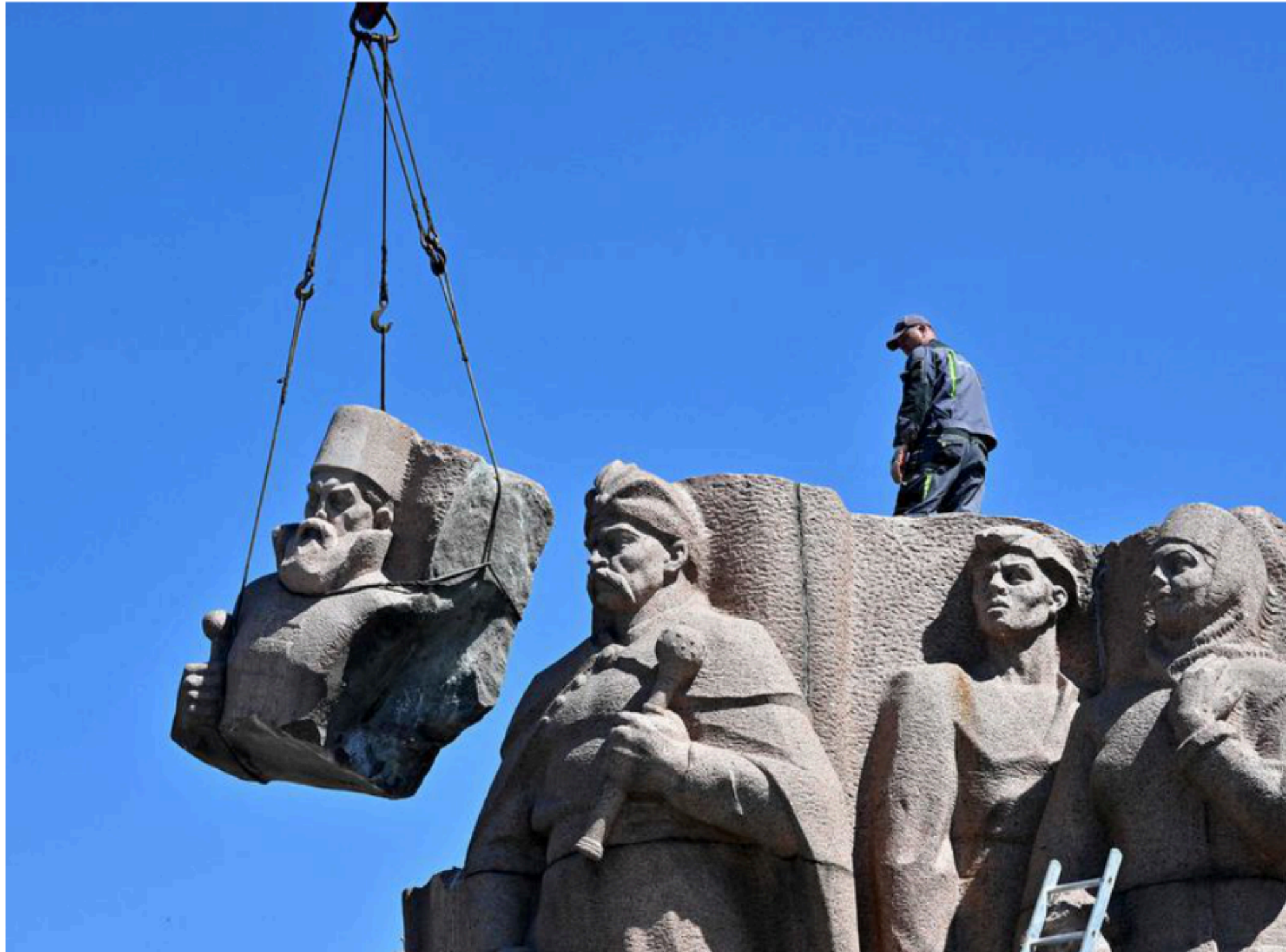
Demolition drive: Workers dismantle a Soviet-era monument to the Pereiaslav Agreement on Ukraine-Russia union, in Kyiv on Tuesday. AFP
